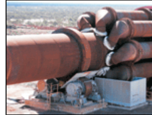
The old refractory lining of Windimurra's 126-metre-long rotary kiln has been removed and its replacement put out to tender.
